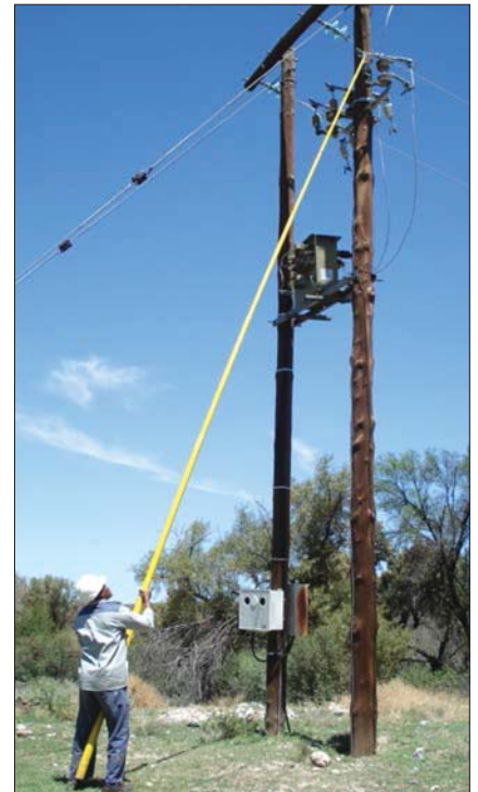
Fig. 5: Surge arrester being replaced live line via a conventional telescopic link stick.
