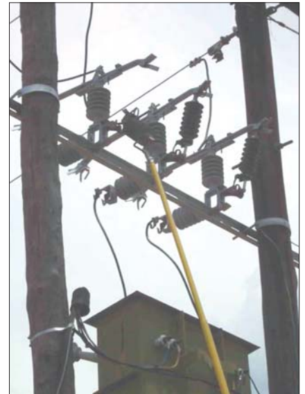
Fig. 4: The live line surge arrester in the Combi unit is positioned not further than 1 m from the transformer, as per Eskom specification, D-DT-1877 & D-DT-1876.
