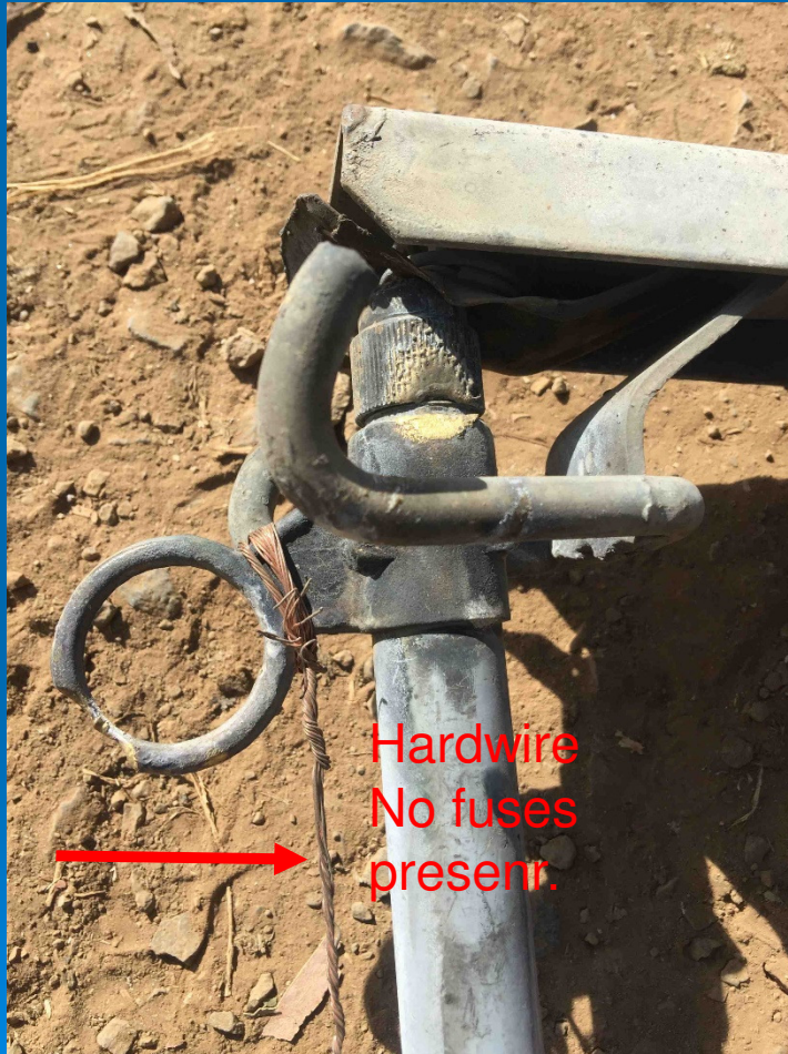
All fuses were blown
