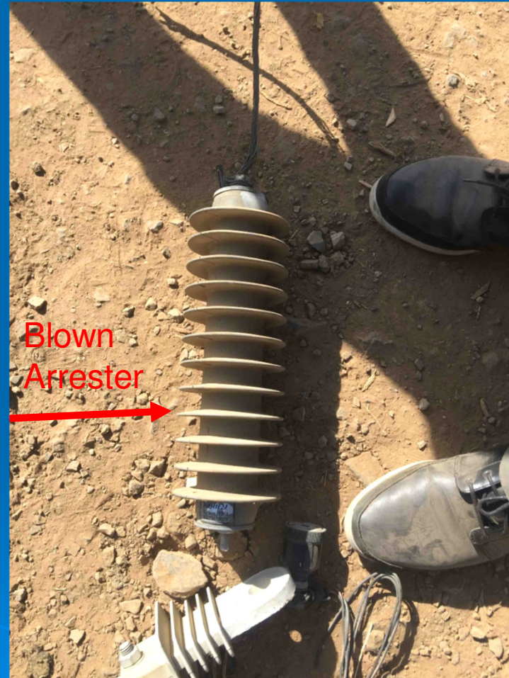
All surge arresters were blown
