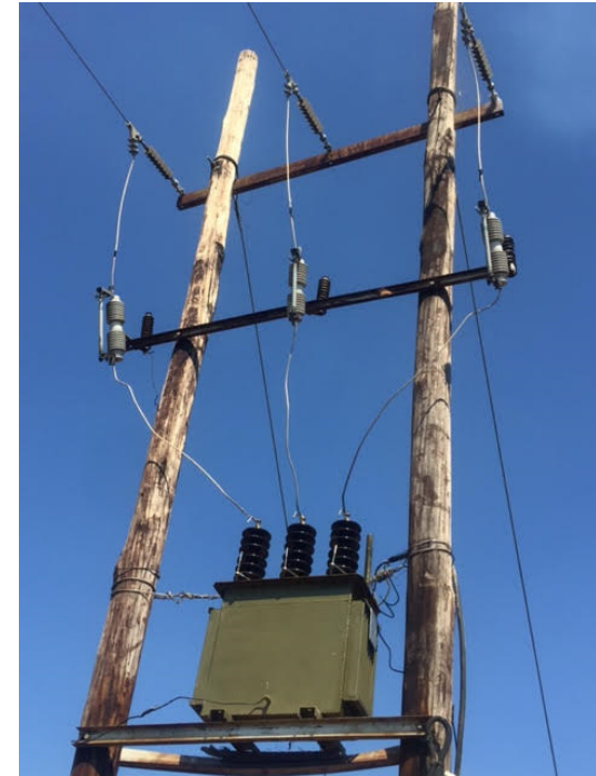
Ndola – Dingaon Xfr 33kv
